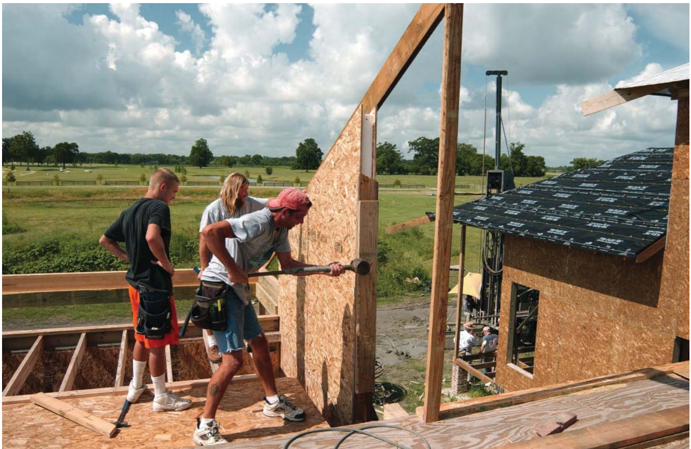
A structural insulated panel system – or SIPS – is featured in LaHouse to create an airtight, insulated attic.
